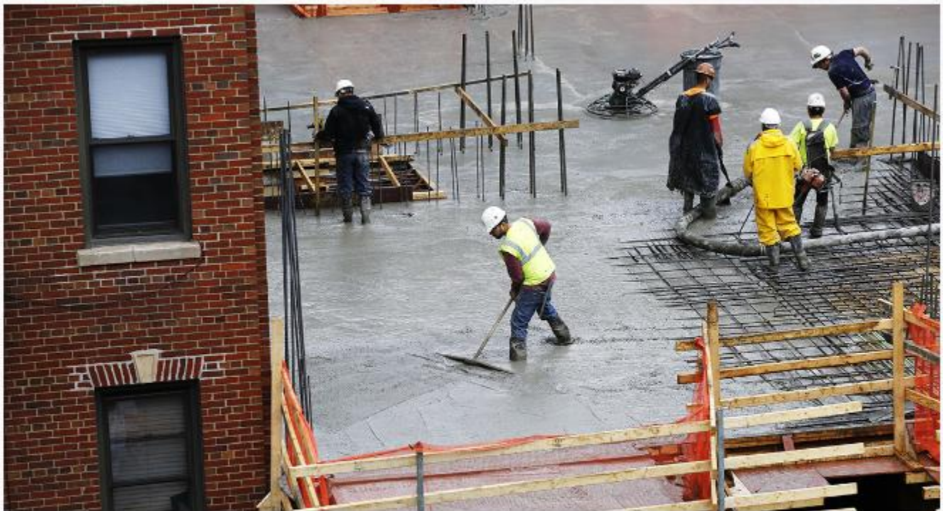
Construction workers smooth wet concrete into place at the site of a new apartment building. | AP Photo/Mark Lennihan
